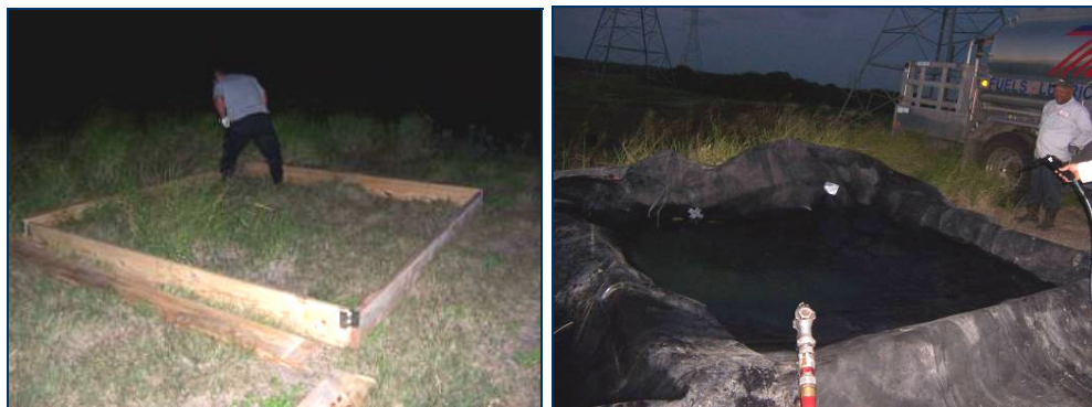
Fig. 8. Ground images showing the construction (left) and filling (right) of 10 x 10' gasoline target prior to overflight at Test Site #1.
